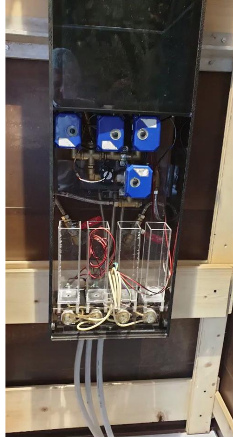
Fig. 7b. View of the valves and dispenser system.
