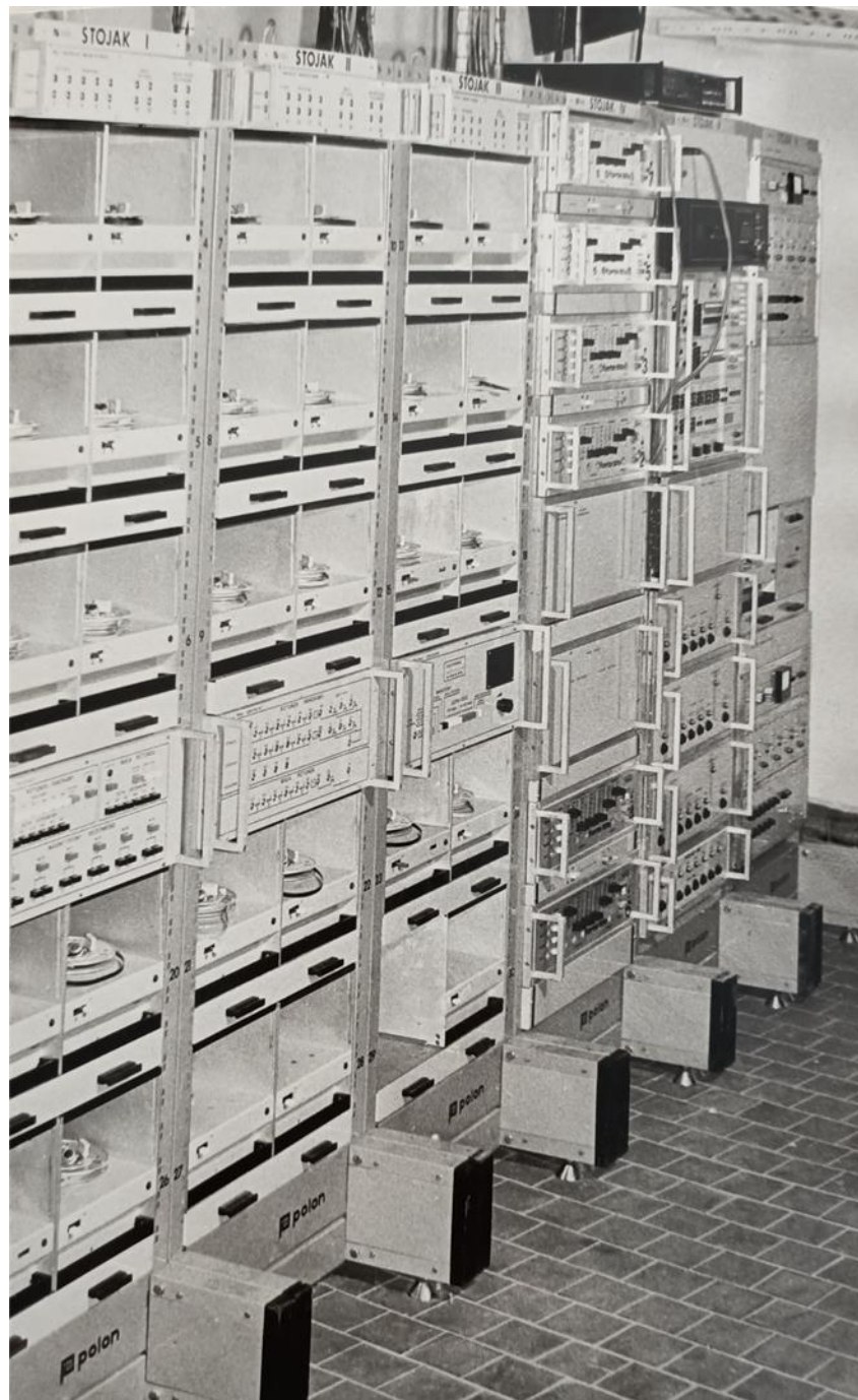
Fig. 9. Amplifiers room – general view of the electroacoustic system equipment on the day of opening of the “Panorama Raławicka” (14 June, 1985)
